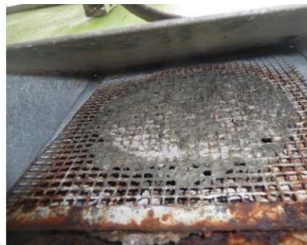
Dirty outdoor air intake.
