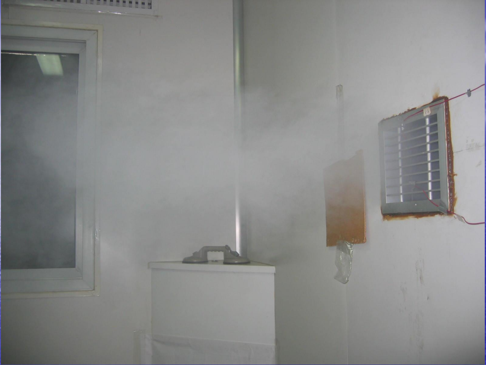
Air supply stratum formed under cooling condition
