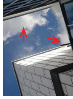
Figure 19: Excessive smoke exfiltration was clearly visible at the top portion of the CW assembly.
