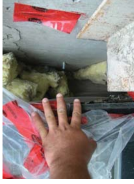
Figure 29: Close-up view of figure 28 - no air seal at the interface detail (the polyethylene sheet was installed as a temporary measure after removing the masonry).
