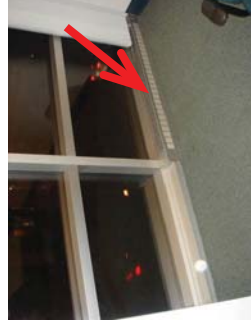
Figure 3: An interior heat source located directly against the interior side of the CW assembly yields misleading results.
