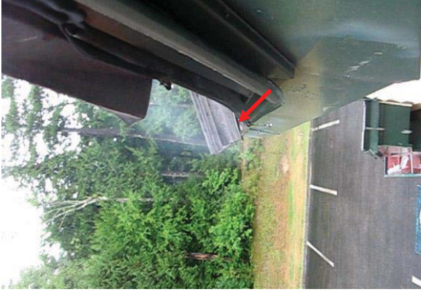
Photo 3: Tracer smoke exfiltration at roof eave (arrow).
