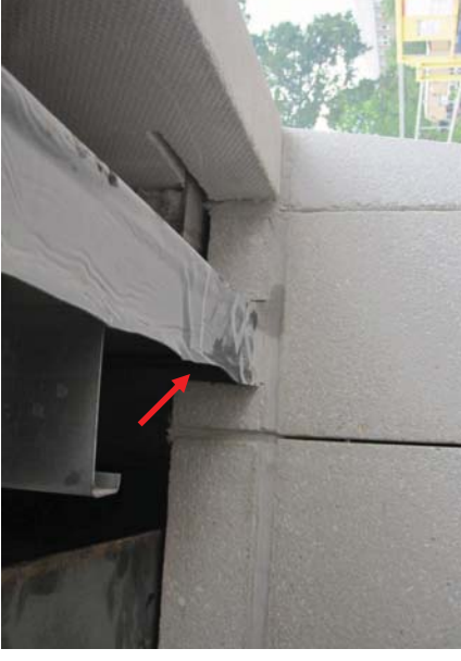
Photo 7: Unsealed beam penetration through air barrier at masonry wall (arrow).
