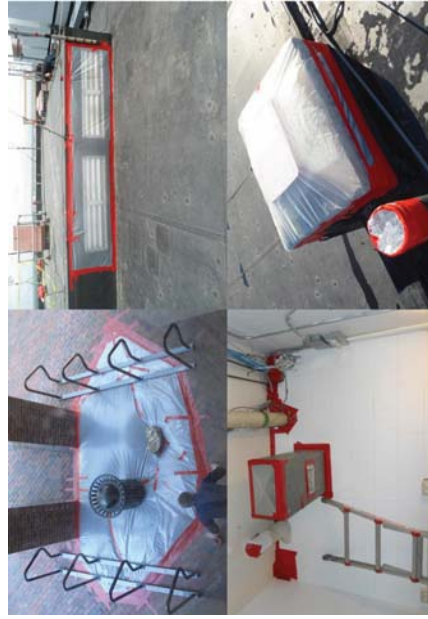
Photo 9: Various envelope penetrations sealed with tape and polyethylene sheet.
