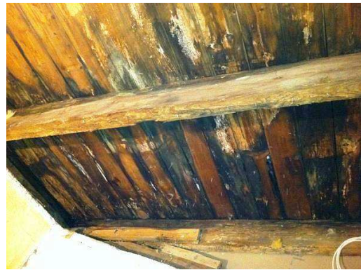
(b) Rot in roof construction due to poor design and inadequate ventilation. Foto © Finn AS
