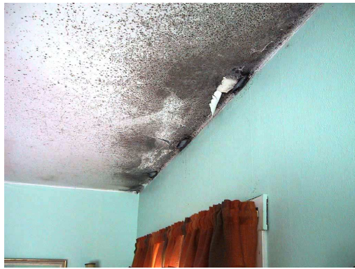
(a) Mold in a naturally ventilated dwelling with poor ventilation. Foto © SINTEF
