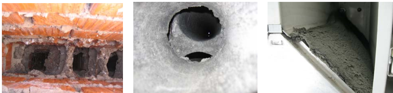
Figure 2: The installation quality of old ventilation shafts is bad (left and middle) and filters of modern ventilation unit have become dirty (right).
