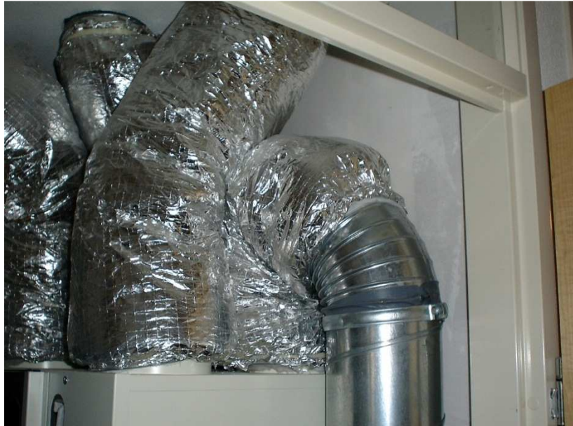
Figure 5: Poorly working system due to incorrect use of flexible connectors
