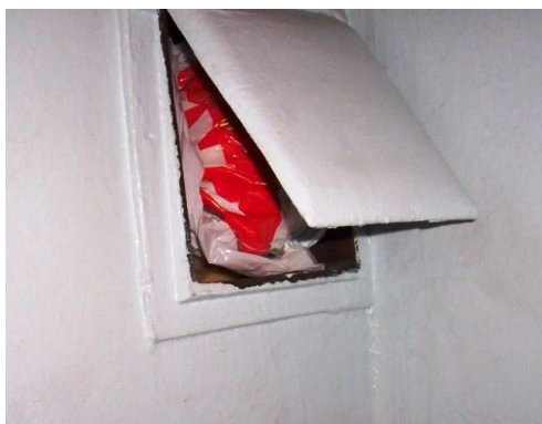
(a) Vents are often closed or blocked to prevent cold drafts and reduce heating costs.
