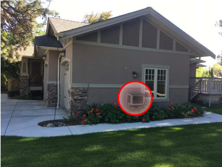
Figure Five: Outdoor air inlet box and filter housing (circled) – case study house
