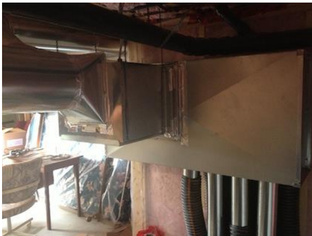
Figure Nine: Ductwork header connected to earth tubes and fan unit.
