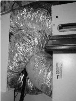
Figure 5 | Example of incorrectly placed flexible ductwork near the ventilation unit.
