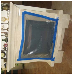
Figure 4. The example of leakiness in the building
