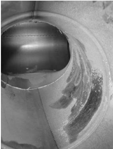
Figure 4 Example of dust accumulation in an air supply duct of a MVHR system.
