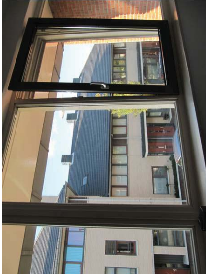
Figure 1. tilted window on first floor under the overhang.
