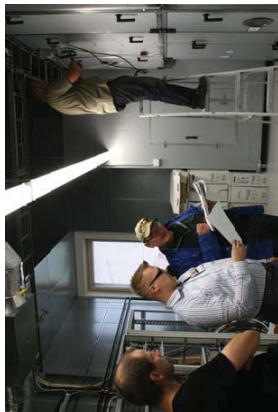
Figure 14. Measurements over the exhaust fan
