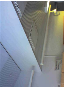
Figure 1. Ventilation duct, inlet to the library
