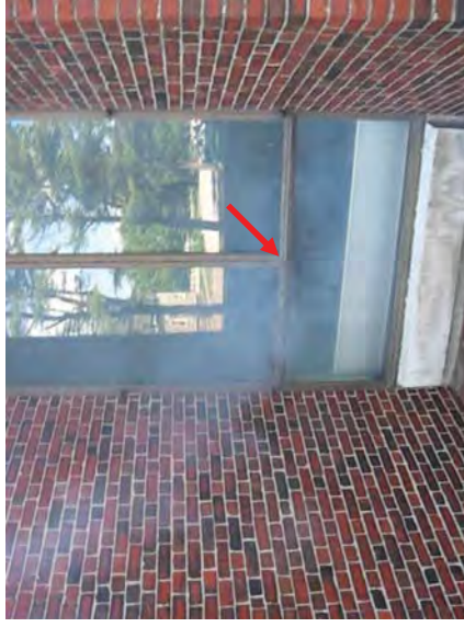
Photo 10: Tracer smoke exfiltration (arrow) at the operable window sash.
