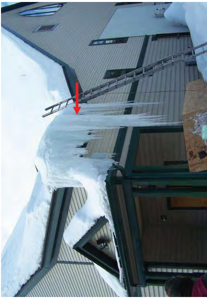
Photo 1: Severe icicle and ice dam formation at metal roof eave (arrow).
