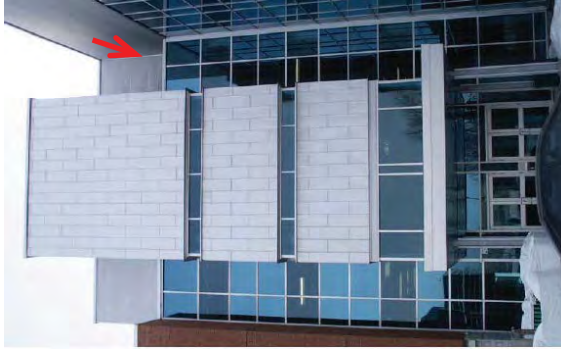
Figure 16: Actual photograph of one of the curtain wall sections inspected for air leakage.
