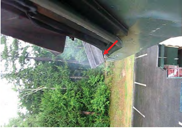
Photo 3: Tracer smoke exfiltration at roof eave (arrow).
