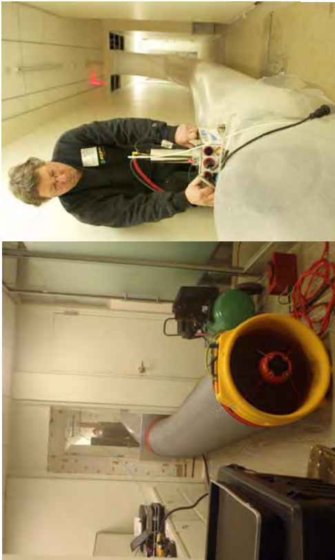
Figure 2: Blower-door fan being applied in combination with the aerosol sealing system (Building 8 in Tables 1 and 2)
