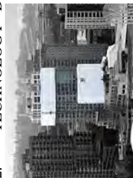
Age: 3 Years. Repair cladding, structural repair, repair windows, new sliding glass doors, project Repair project cost: $13 Million.
