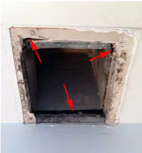
Figure 2 – Gaps between exhaust ductwork and surface mounted grilles (removed in this photograph)
