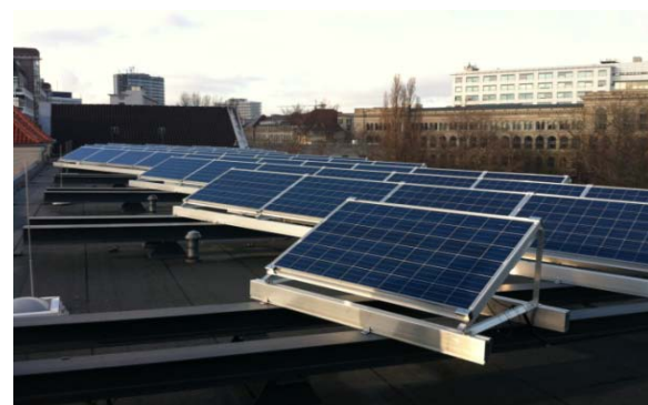
Figure 4 Monitored PV-generator on the roof of the UdK Berlin building Hardenbergstraße 33
